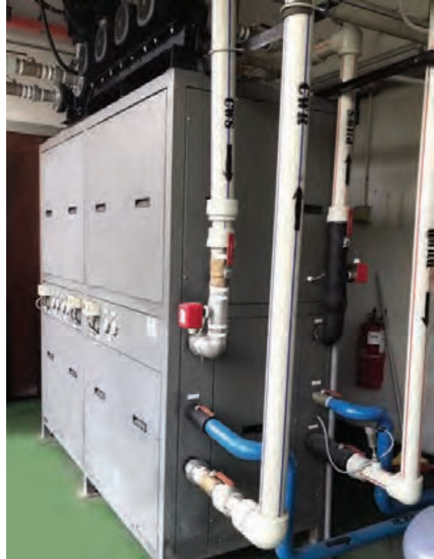
Heat recovery system installed at one of the Group's factories in Malaysia.
