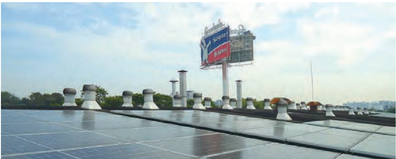
Solar panels installed on the rooftop of one of the factories of our joint venture in Malaysia.
